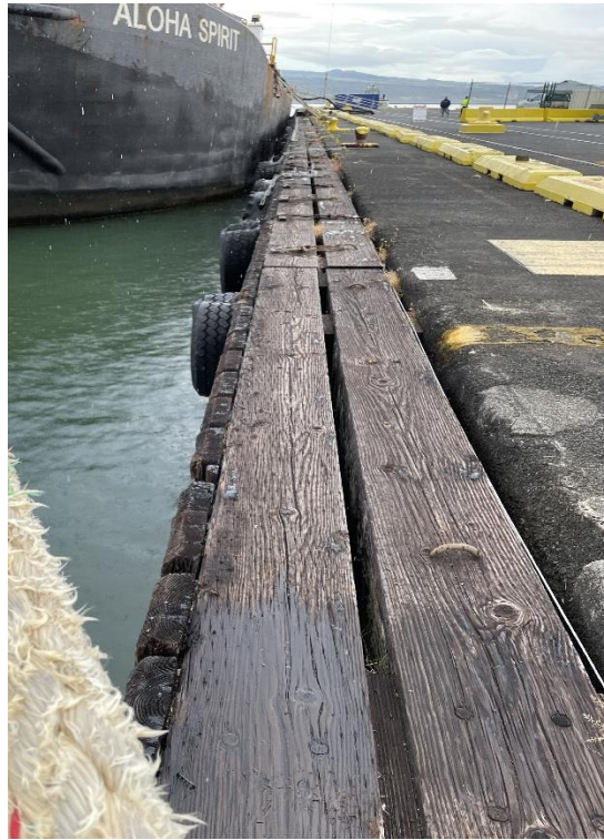
Photo 3: Existing Pier 3 to be repaired. View looking northwest.
