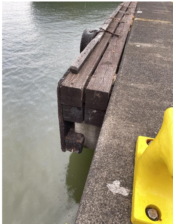
Photo 2: Existing Pier 3 to be repaired. View looking northwest.
